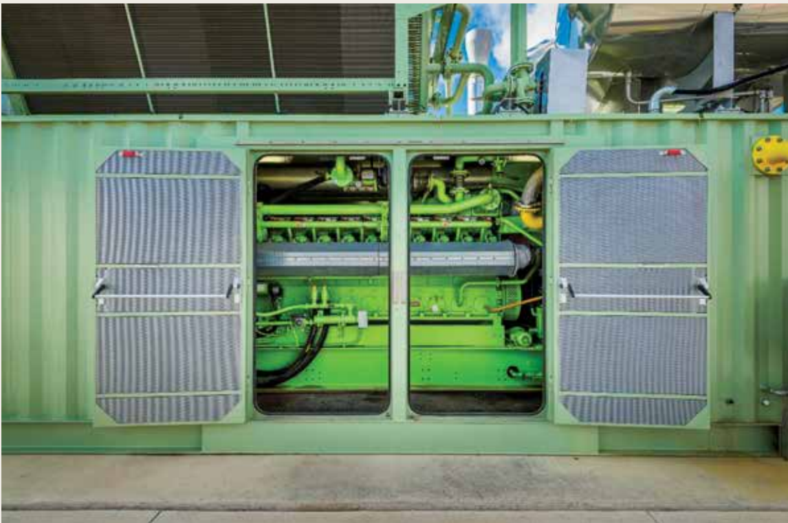
LMS Energy's Seaford Bioenergy Facility, South Australia.
